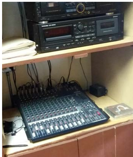
Current sound board to be tied in to new recording system
